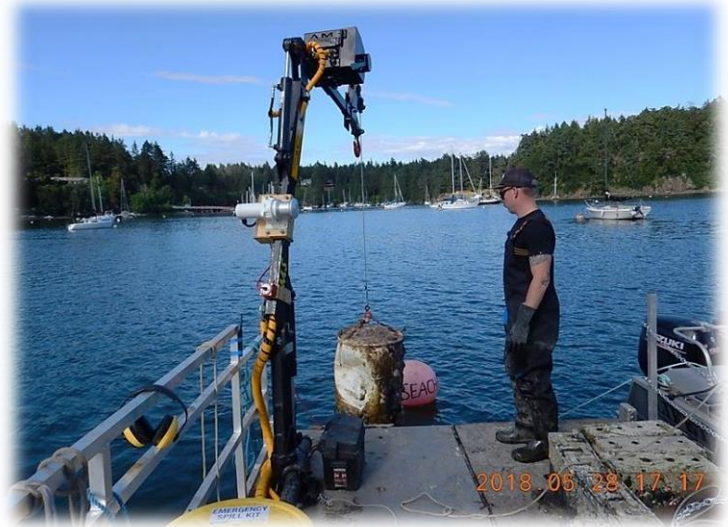
Raising debris from the seabed of Degnen Bay with the crane on the SeaChange boat, Collective Effort .
